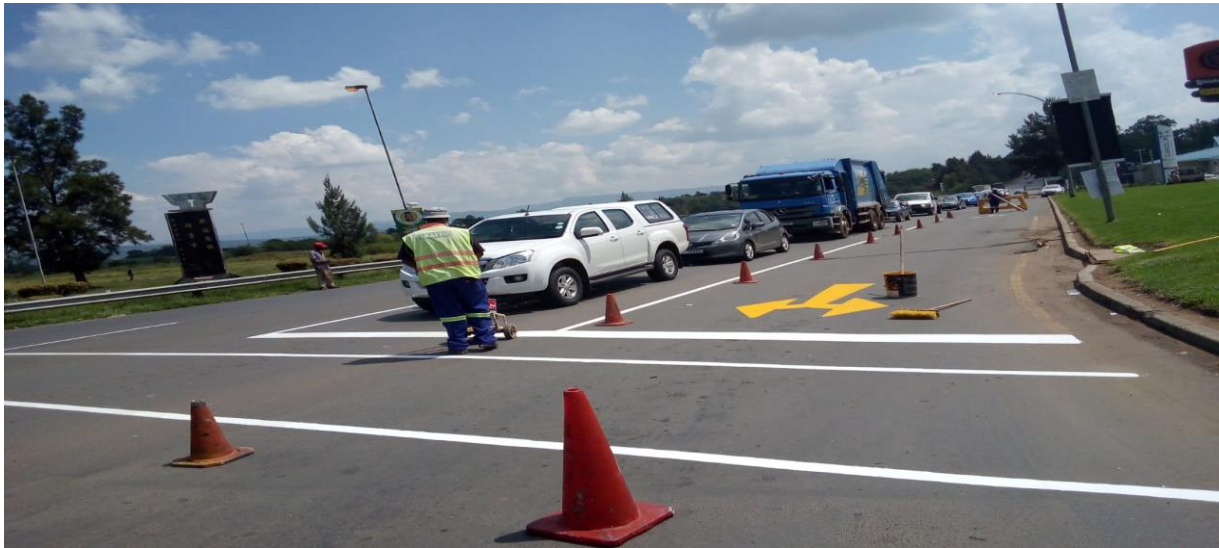
Road marking team from Community Safety busy at the intersection of Allen Street and Memel Road.
