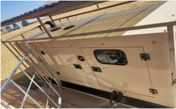
Figure 20 Generator installed at Charlestown Library
