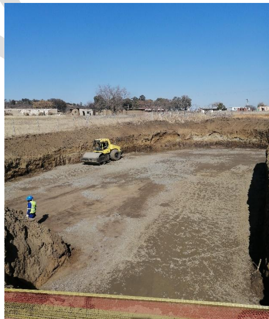
Additional 500Kl balancing reservoir
