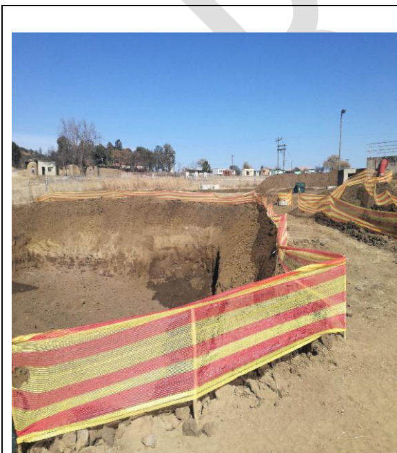
Additional 500Kl balancing reservoir
